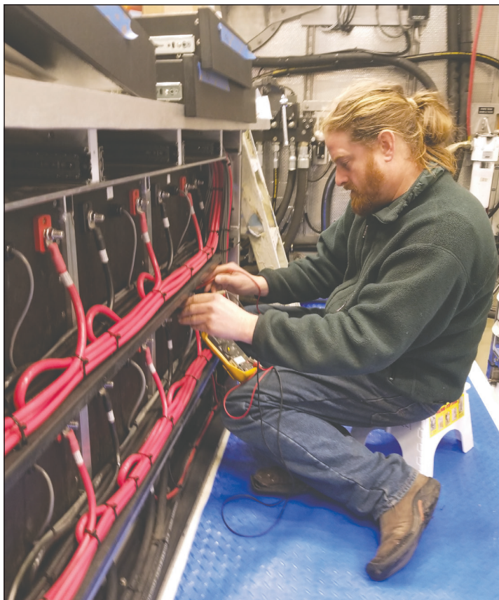
Revision Marine LLC co-founder Matt Mortensen tests their large format lithium batteries installed on the 92-foot expedition vessel New Pacific . Courtesy of Revision Marine LLC.
